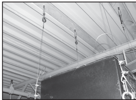
Fig. 15: Eyebolts in place of threaded rod.
